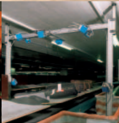
Reading systems with 10 CLV490 barcode readers and an OTC evaluation unit each are installed above a case sorter and identify the flight baggage.
